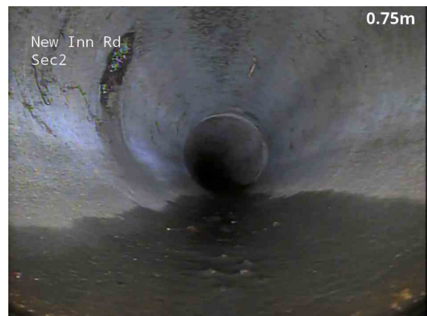
4, 00:00:09, 0.90 m Fractures, multiple from 12 o'clock to 12 o'clock, finish
