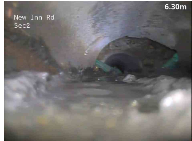
8, 00:01:12, 6.40 m Settled deposits, coarse, 40% cross-sectional area loss, change
