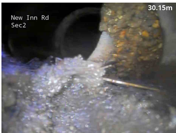
21, 00:04:00, 30.40 m Survey abandoned, Unable to continue
