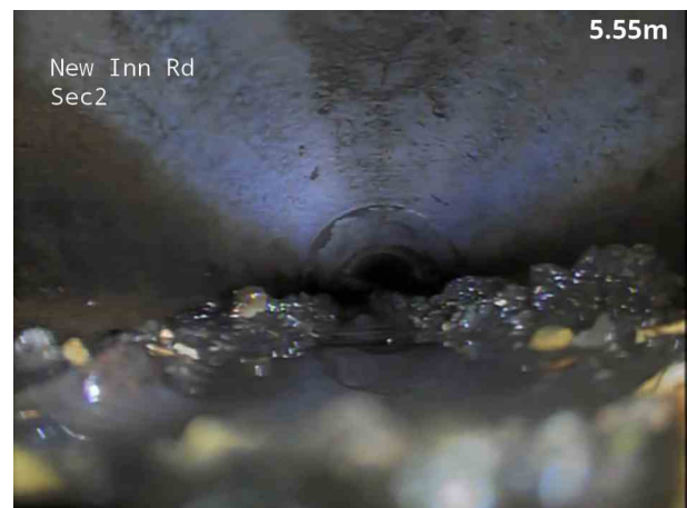
6, 00:00:26, 5.60 m Settled deposits, coarse, 20% cross-sectional area loss, change
