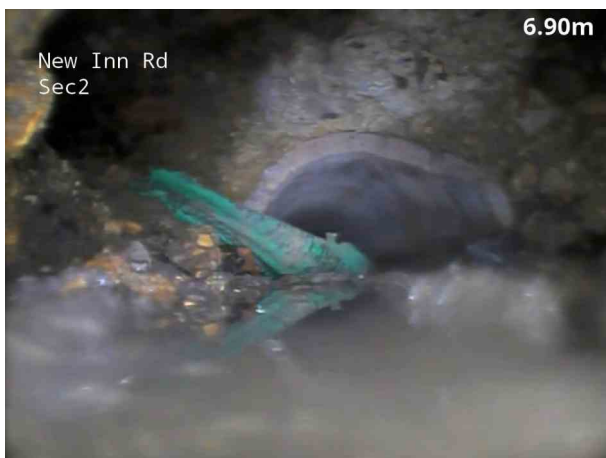
9, 00:01:22, 7.00 m Hole in drain or sewer from 8 o'clock to 4 o'clock, start
