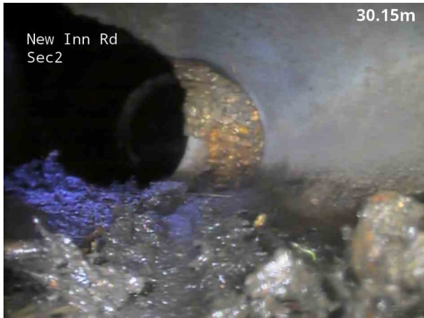
19, 00:03:34, 30.40 m Broken pipe from 12 o'clock to 4 o'clock
