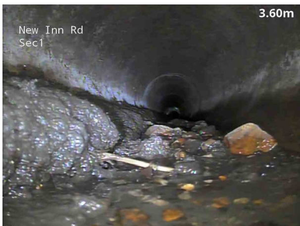
3, 00:00:25, 3.60 m Settled deposits, coarse, 10% cross-sectional area loss, start
