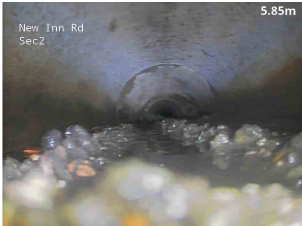
7, 00:00:29, 6.00 m Settled deposits, coarse, 30% cross-sectional area loss, change
