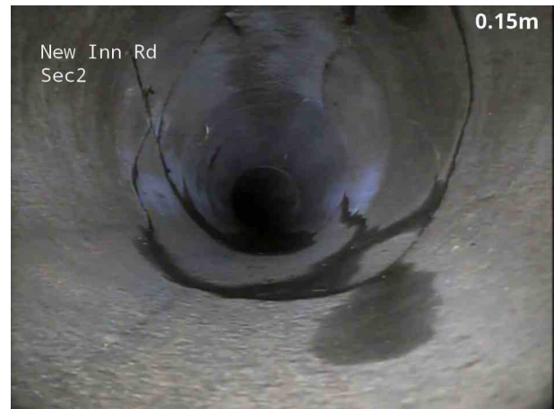
2, 00:00:05, 0.50 m Fractures, multiple from 12 o'clock to 12 o'clock, start
