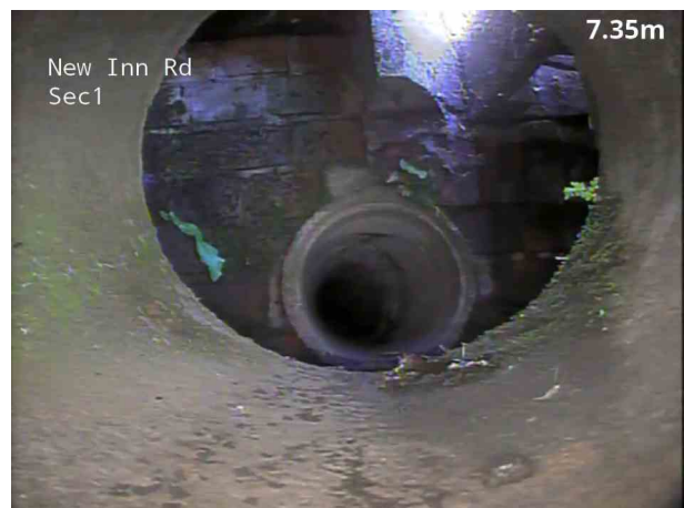
4, 00:00:48, 7.30 m Settled deposits, coarse, 10% cross-sectional area loss, finish
