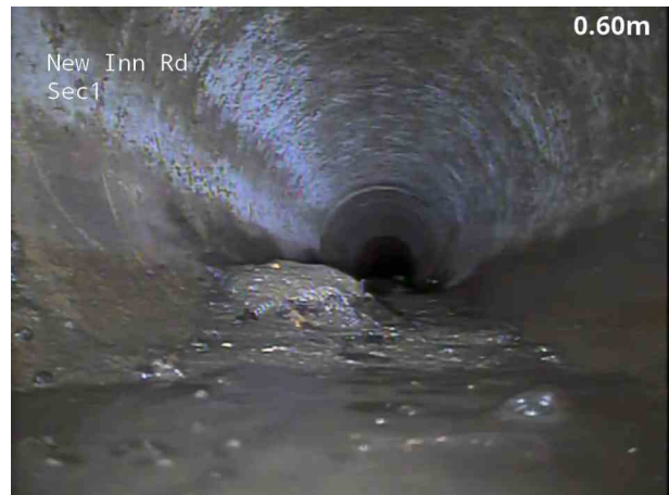
2, 00:00:08, 0.80 m Settled deposits, fine, 10% cross-sectional area loss, start
