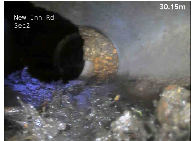
20, 00:03:35, 30.40 m Line deviates right, Junction with unknown
