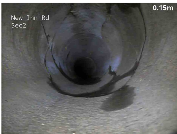
3, 00:00:05, 0.50 m Fractures, multiple from 12 o'clock to 12 o'clock, start
