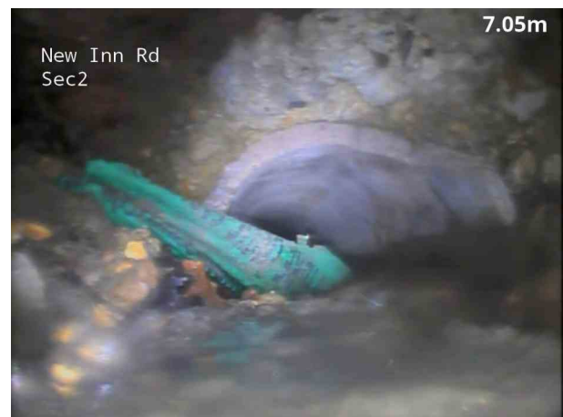
10, 00:01:22, 7.00 m Hole in drain or sewer from 8 o'clock to 4 o'clock, start
