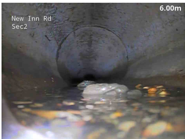
5, 00:00:23, 5.00 m Settled deposits, coarse, 10% cross-sectional area loss, start
