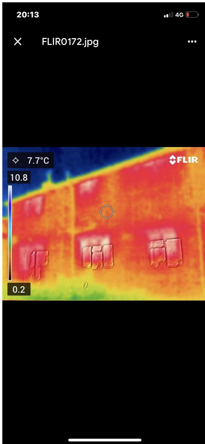
Thermal Camera Image of a Property Feb 2023
