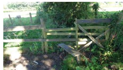
Broken Stile at eastern end
