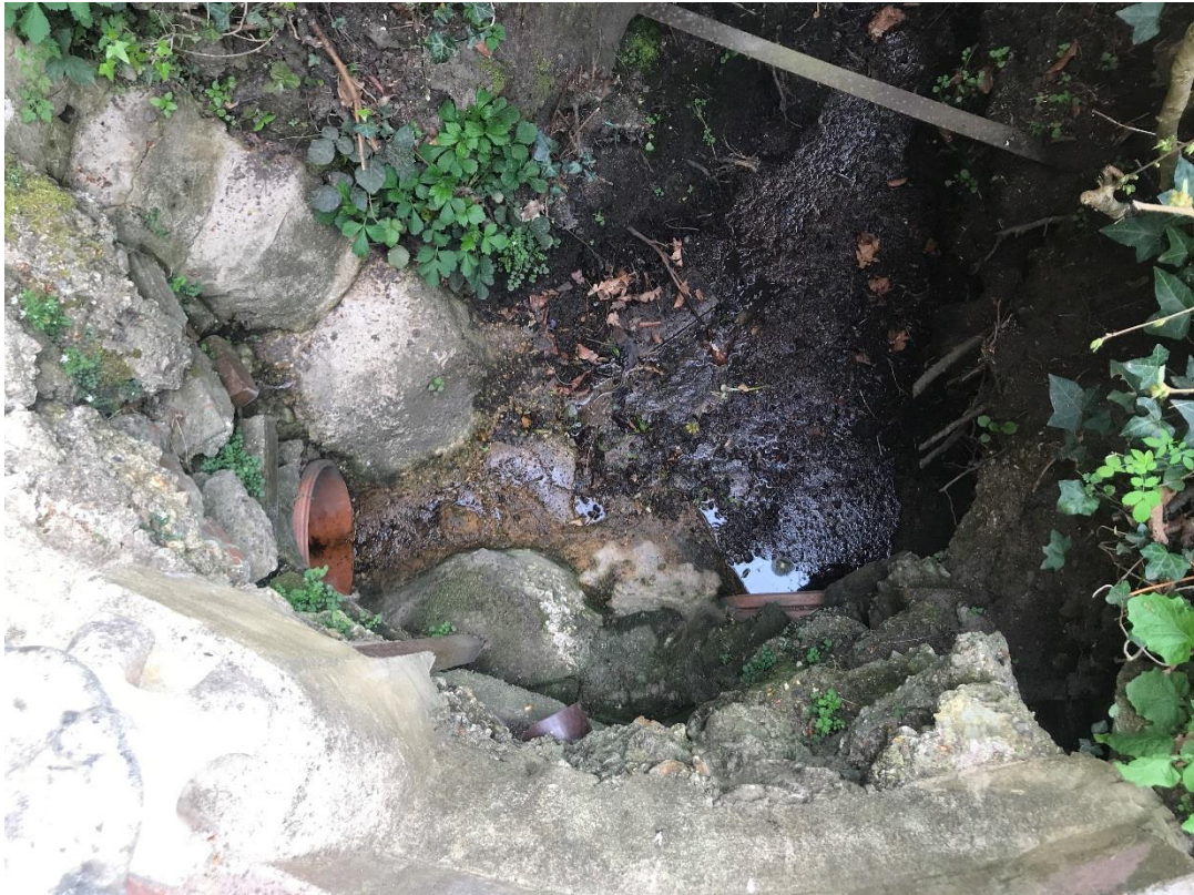
Image 5 : Pipe system under Stanley Cottage, Windsor Road, which joins the open watercourse thought to originate from Spring Cottage (April 2019)
