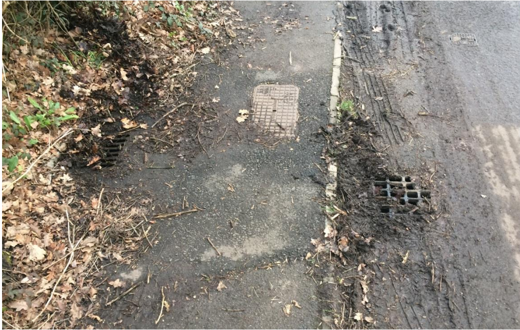
Image 1: Example of current highway drainage on Pollards Moor Road impacted by detritus (Jan 2018)
