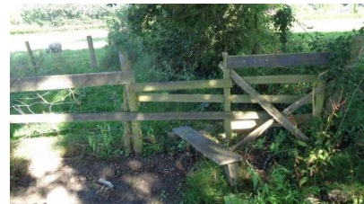
Broken Stile at eastern end
